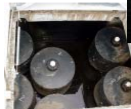
Filters in the vault.
