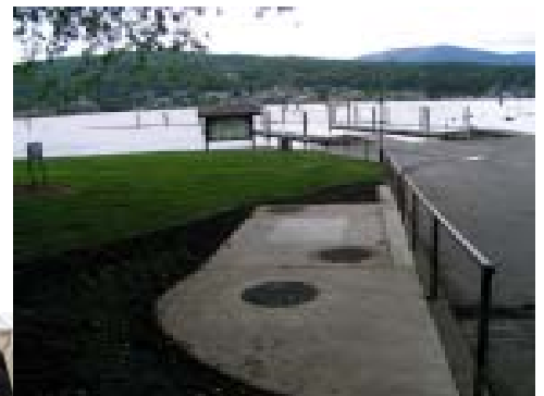
Completed StormFilter® system.
