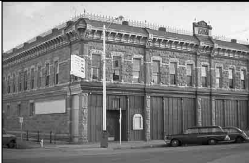
The windows in this building were boarded and architectural details needed repair. (Compare with the photo below).
