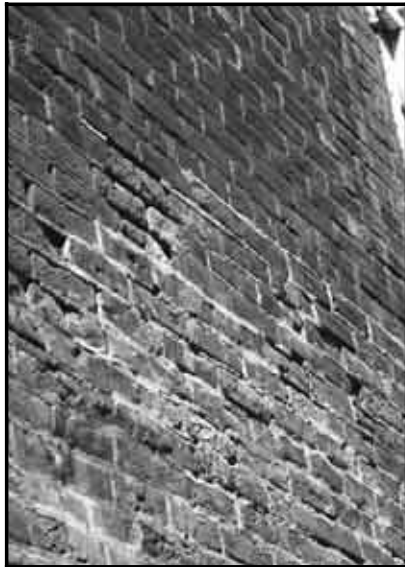
Protect masonry from water deterioration.
