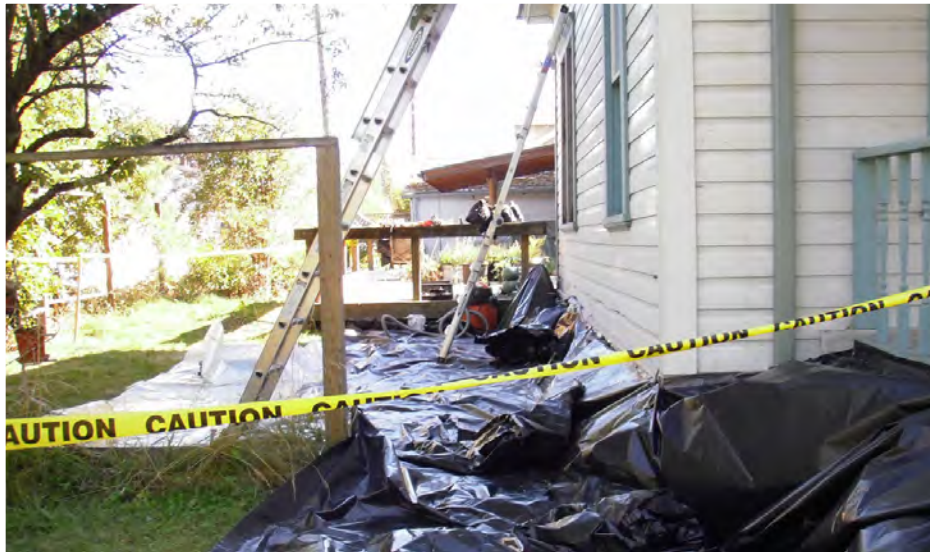
Repainting Home with Lead-Based Paint
